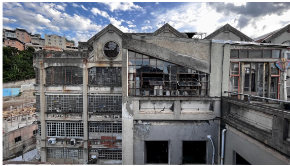
Fig.3 - Bhering Factory in poor condition of preservation.
